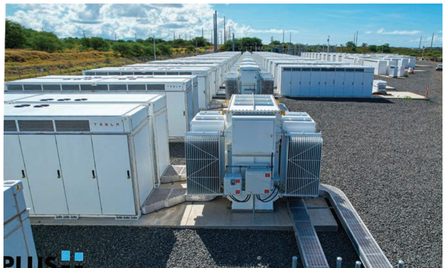
The battery storage project at Kapolei Energy Storage (KES) has the capacity to power 20% of O’ahu’s energy needs. PHOTO COURTESY OF KES
